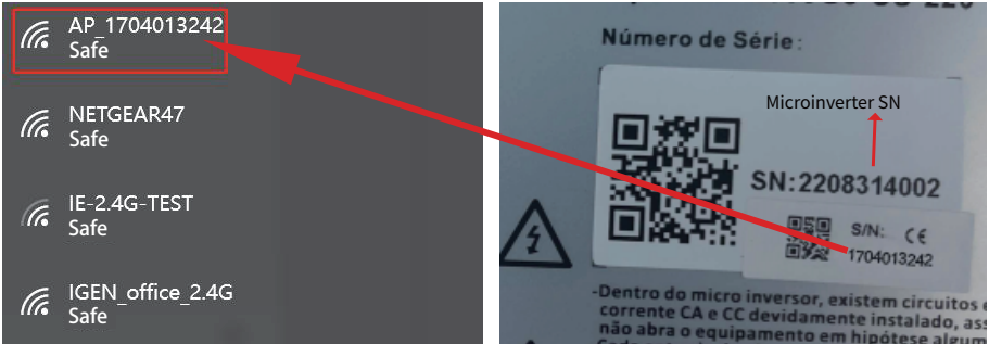
Microinverter SN: 2208314002 Built-in datalogger :1704013242
